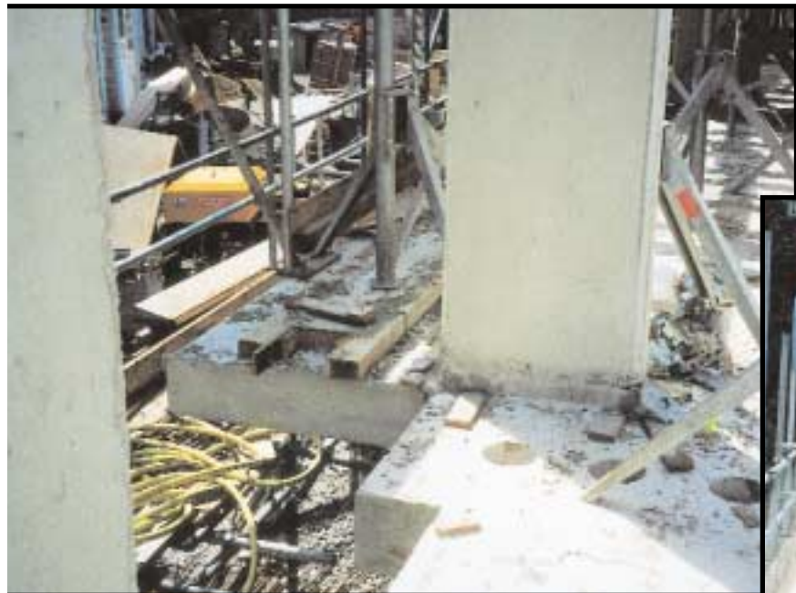
This unprotected gap in a floor was one example of failure to prevent the risk of falls from height which led to work being stopped at this site in Camden.
