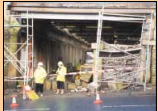
This stone archway collapsed because demolition work was not done properly
