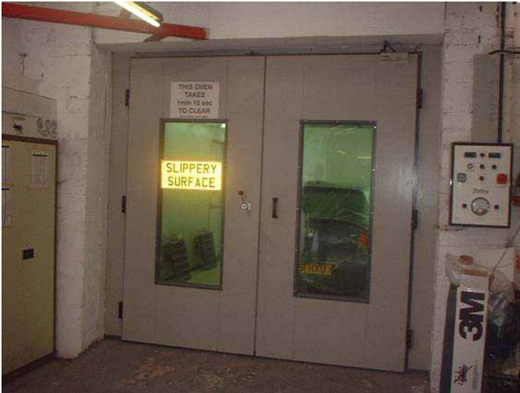
Photograph 1: Clearance time displayed on booth doors
